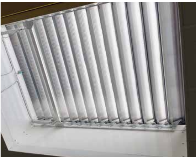
Fig. 39 – mcr LAM louvered vent, roof mounted - inside view
