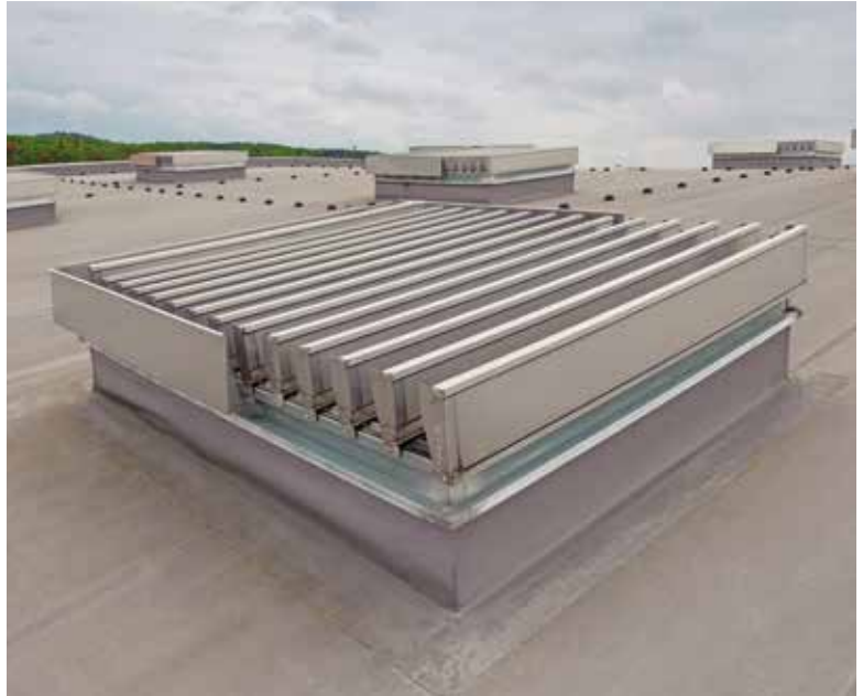
Fig. 37 – mcr LAM louvered vent, roof mounted
